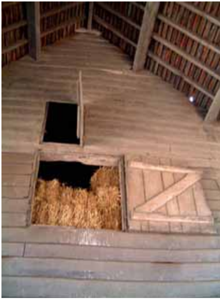
Manor farm south barn, original wide board cladding and loading hatches in the midstrey
